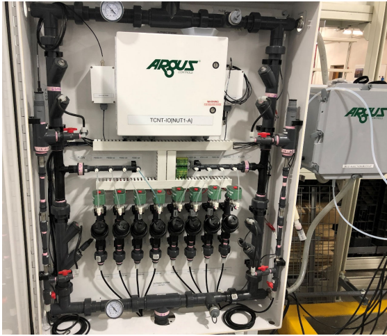
Eight injector system
